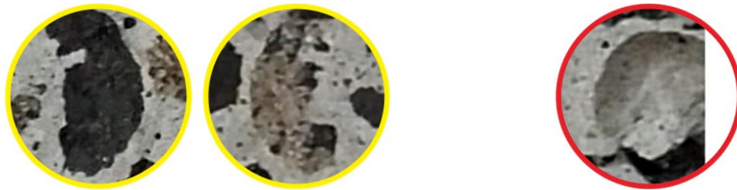
a) Aggregate surface fracture
