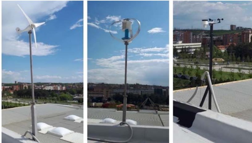
Figure 4 HAWT (left), VAWT (middle), and MWS (right) installed in the rooftop of the Laboratory building of the Technical Faculties of the University of Prishtina "HASAN PRISHTINA"
