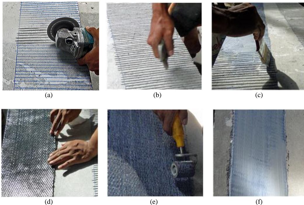
Figure 4 FRP application: (a) surface preparation; (b) sand blasting; (c) first epoxy layer; (d) FRP application; (e) attaching treatment; (f) final epoxy layer
